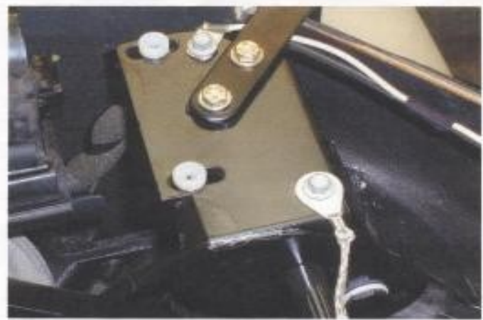
Fig:3 Showing larger piece of angle iron correctly bolted to steel plate by 6 mm bolts and nuts (underside) (Driver's side)
